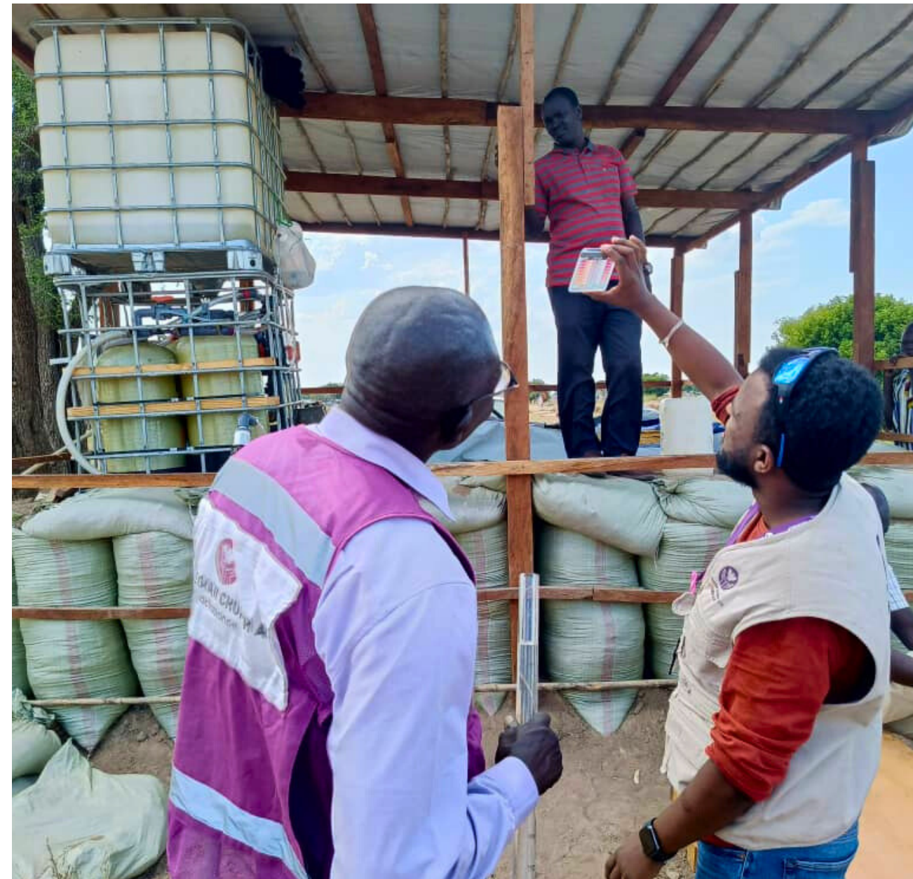
Secure water treatment system (SWAT) constructed to filter surface water
